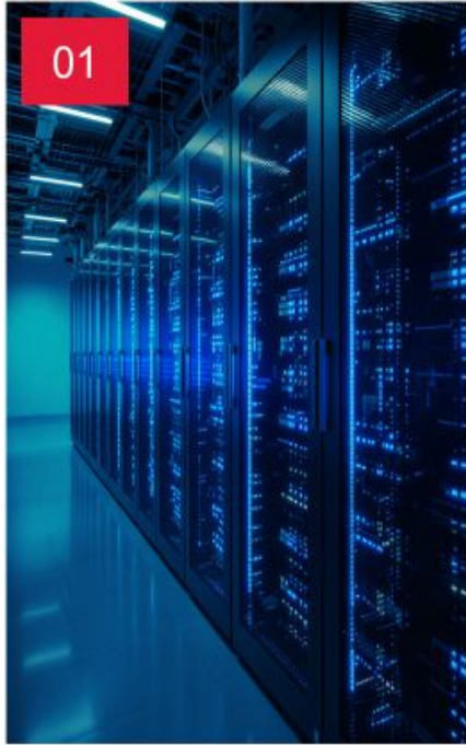
Data Centers AWS, AI Infrastructure
